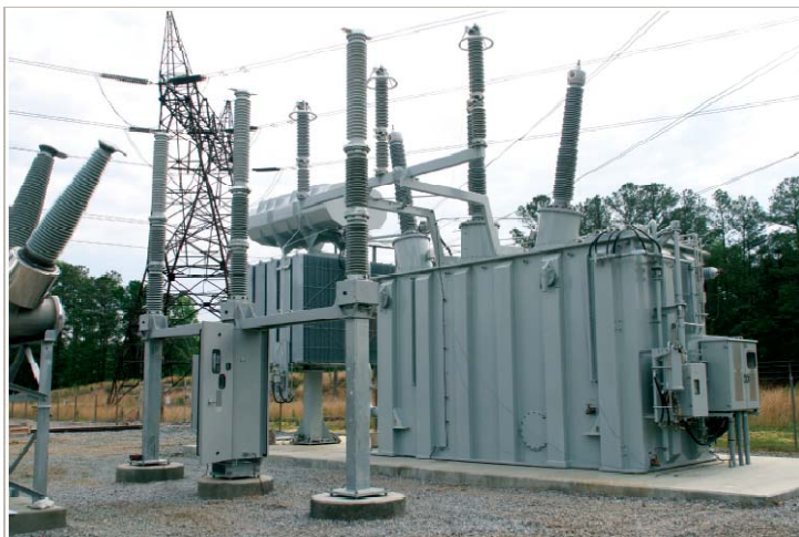
Fig. 6. 230 kV Special purpose shunt reactor switch
