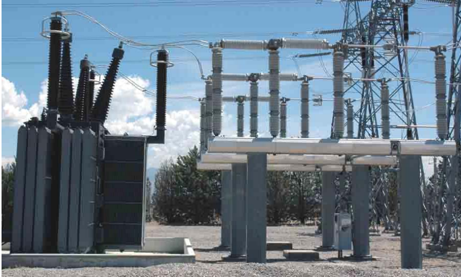
Fig. 6. Oil-immersed shunt reactors switched with a circuit breaker (horizontal interrupter)
