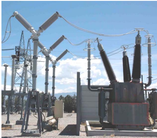
Fig. 4. Shunt reactor switched with a SF 6 breaker
